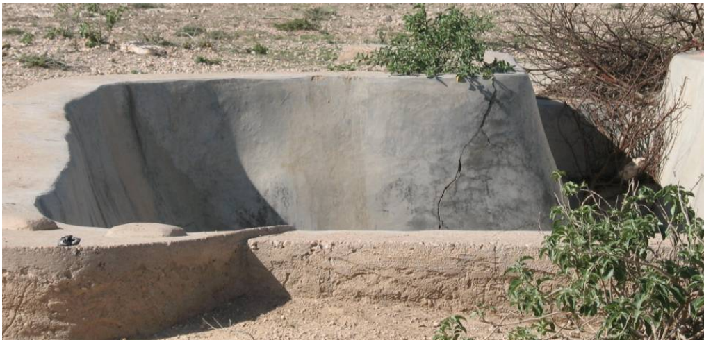
Figure 4.2 Cracks on berkad wall
